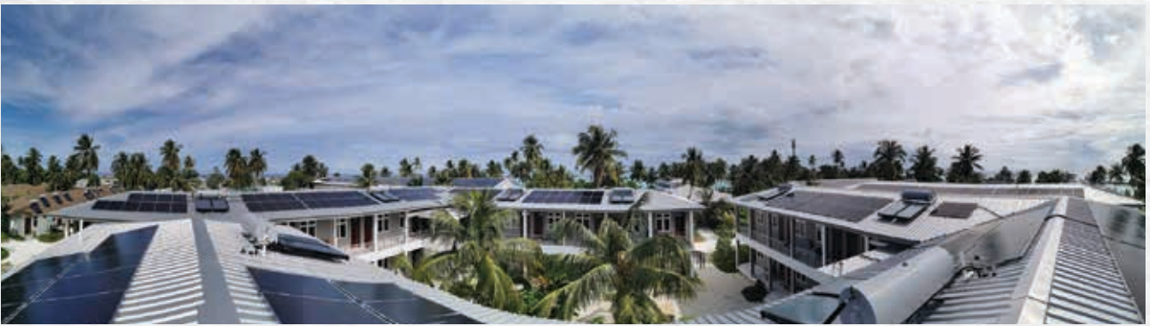
Solar panels installed at the Pullman Maldives Maamutaa Resort
