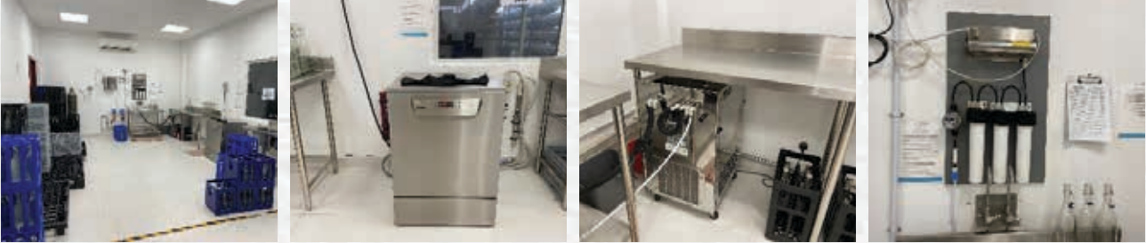
Bottling room, bottle washer, water cooling system and mineral filters (left to right)
